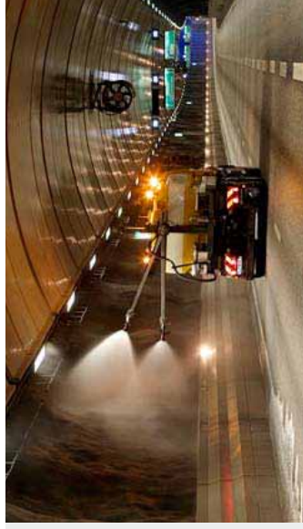
The cleaning of the walls and ceiling is performed under low pressure (8-10 bars) and large quantities of water (some 700 litres/min).
